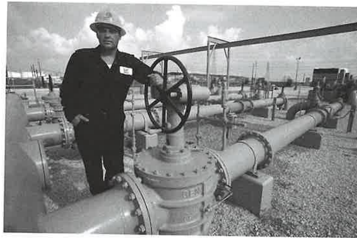
FIGURE 1.2 Clint A. Brist is an operator for Colonial Pipeline in Houston. The facility is a starting point for delivery of petroleum products along 5500 mi of the pipeline. (Courtesy of Colonial Pipeline Company; photograph by Robin Hood.)
