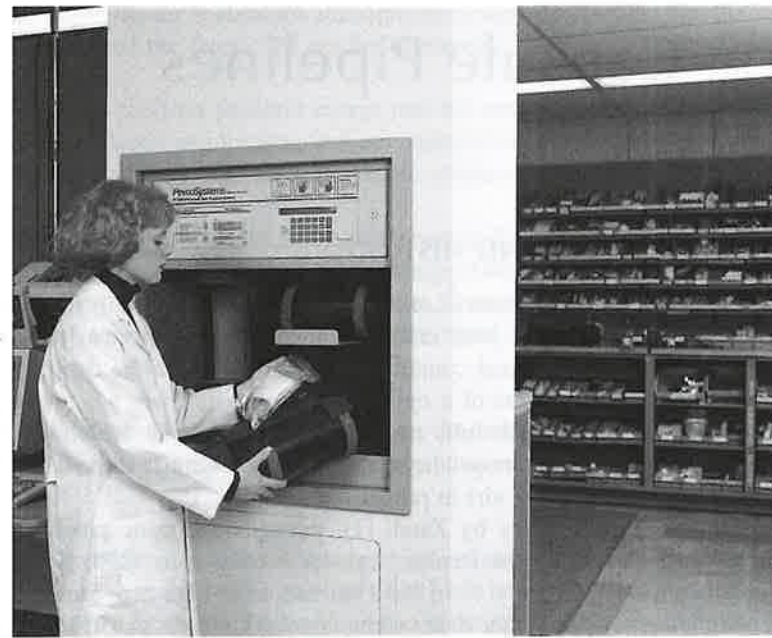
FIGURE 7.1 PEVCO's computerized PCP (pneumatic tube) system used at the Johns Hopkins Bayview Medical Center in Baltimore, Maryland, U.S.A. (Courtesy of PEVCO.)
