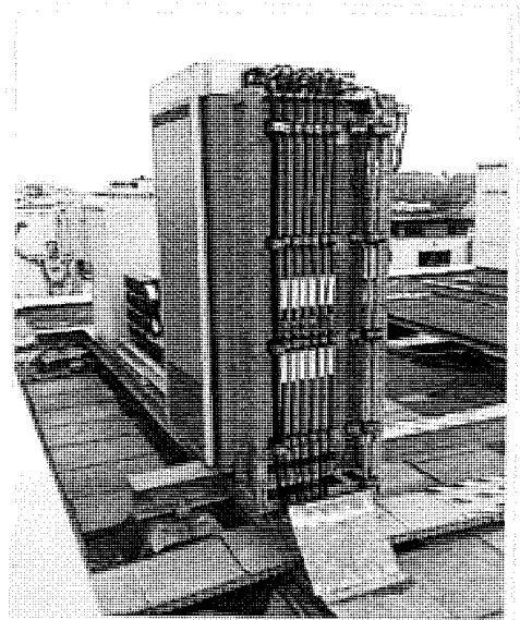
UMTS base station on the roof of a building
