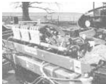
System makes use of a Red Ball monitor which consists of clear plastic tubes with balls floating in them. They tell you at a glance how each row is operating.
