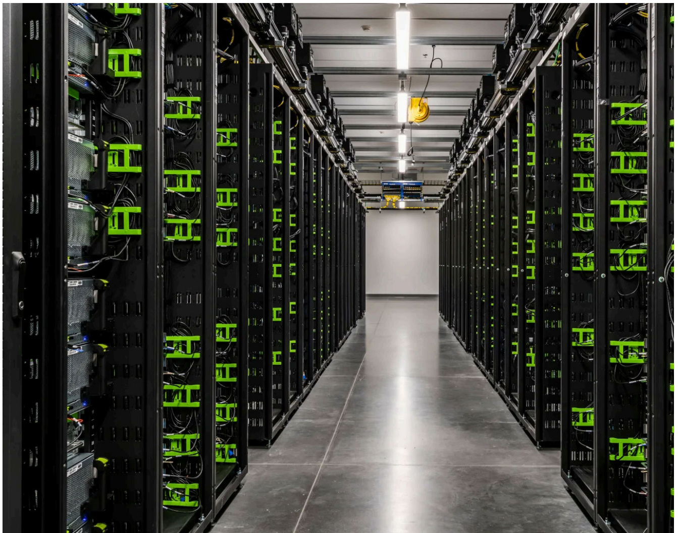
Inside our New Mexico data center.
