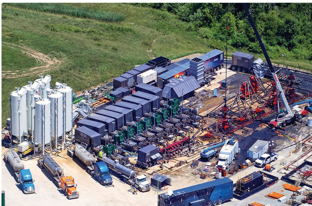
Slim and trim: The electric pressure pumping fleet takes up about a third of the area on a well pad that a conventional fleet of 20-25 pumps normally would, while also incurring far lower fuel costs by utilizing local sources of natural gas. Source: Evolution Well Services.
