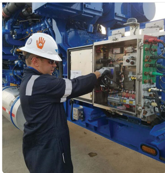
A technician inspects a newly installed after-market control system. Source: IOT-eq.
