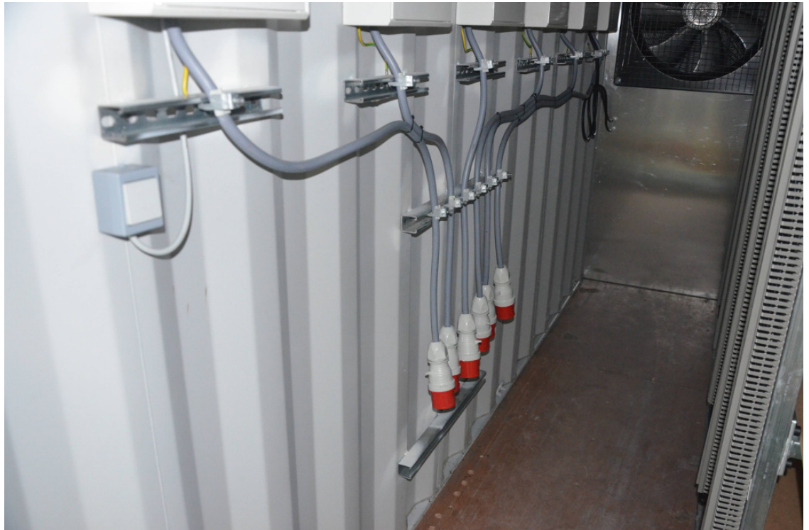
C13 connection cables
