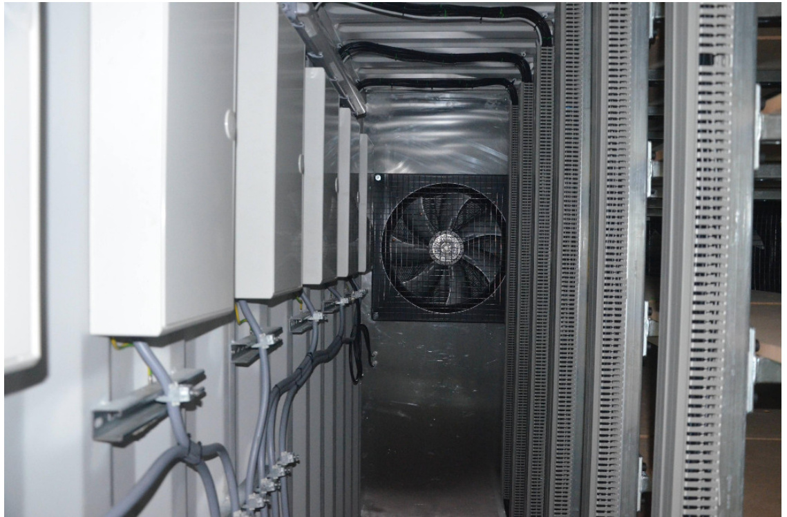
Power distribution box from inside
