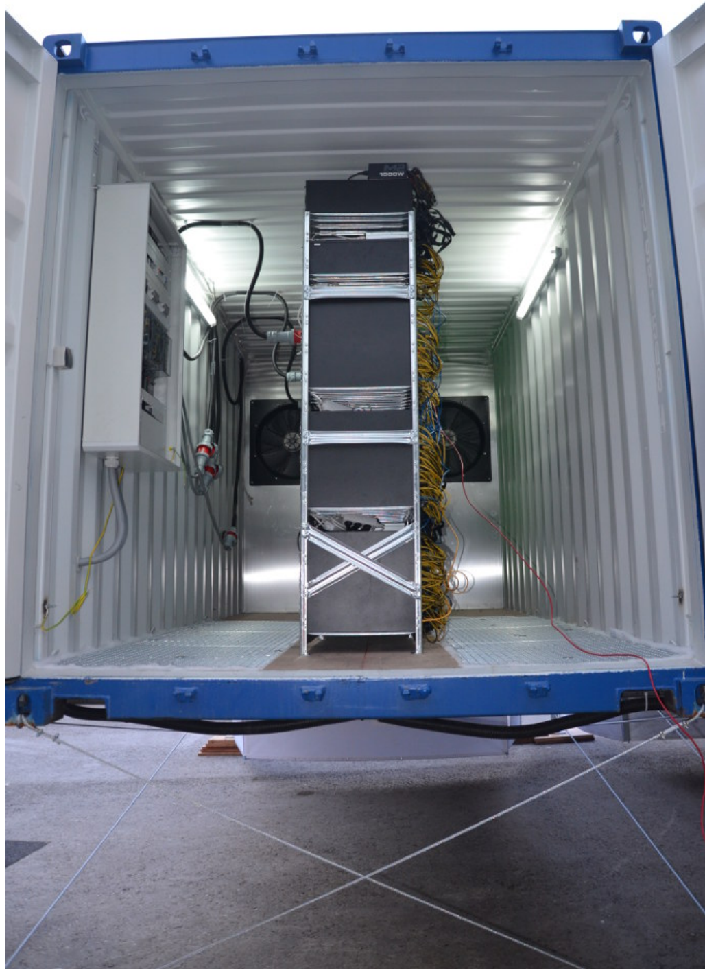
Hot aisle, faster running fan: Cold aisle, slower running fan:
