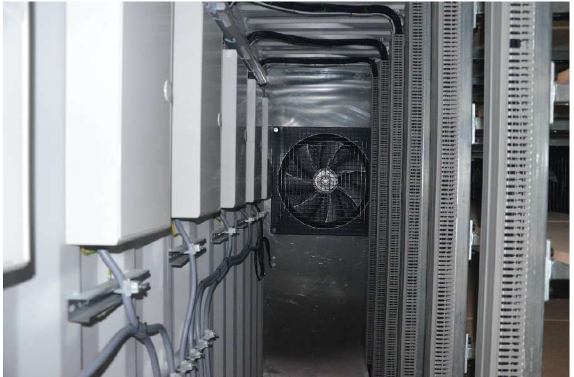
Power distribution box from inside
