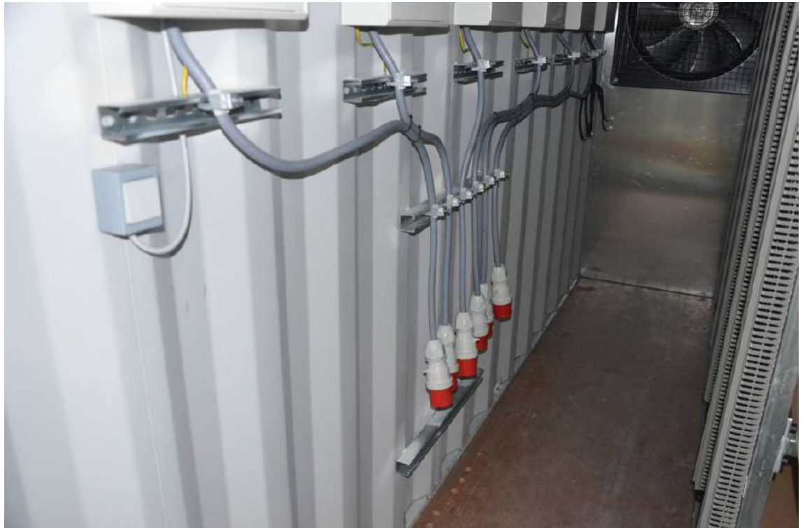
C13 connection cables
