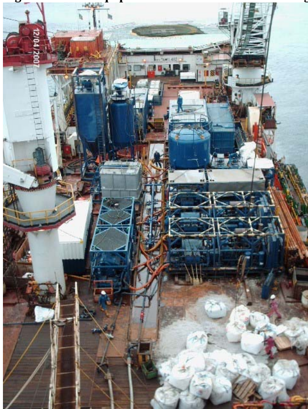
Figure 2 – Frac Equipment on Barracuda Tender Barge
