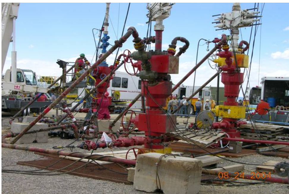
Figure 7: Multi-well simultaneous stimulation operations showing wellhead and piping layout
