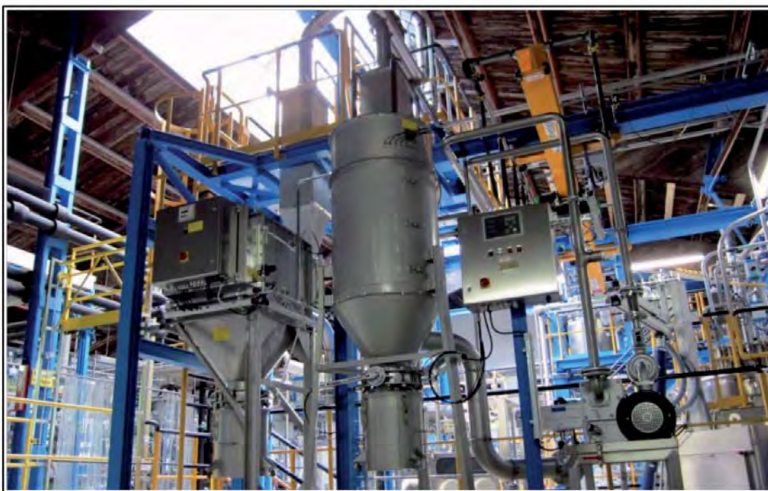
Figure B-32: Solids handling
