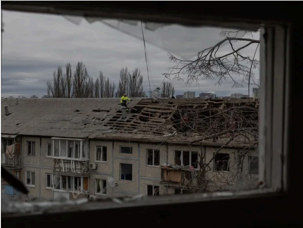
Workers clear debris from the roof of a damaged residential building following a drone strike in Kyiv, on December 23, 2025, amid the Russian invasion of Ukraine. (Roman Pilipey/AFP/Getty Images)
